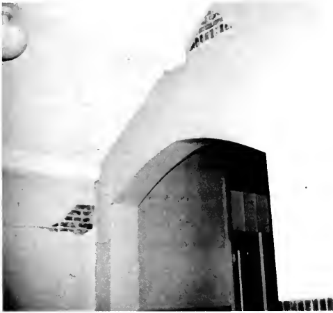
Photo 7. Morningside Elementary School. Unrehabilitated pre-Field Act building. Typical interior-wall damage.
